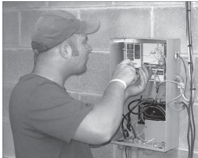
Matt Weiser works on the optical network terminal, where the fiber connects to the customer's home or office.
